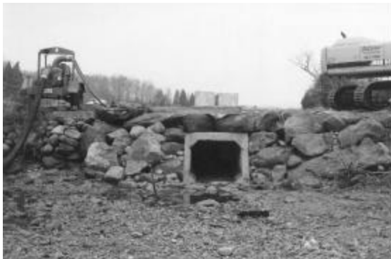
Here's the new culvert shortly after installation, before the tides were let back into the Upper Cove.
